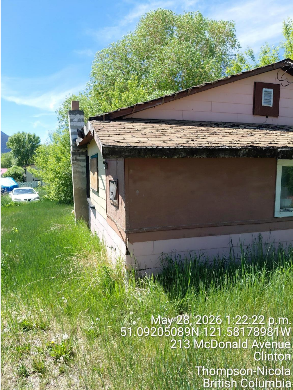
Image showing long grass and broken window with possible access to the home
